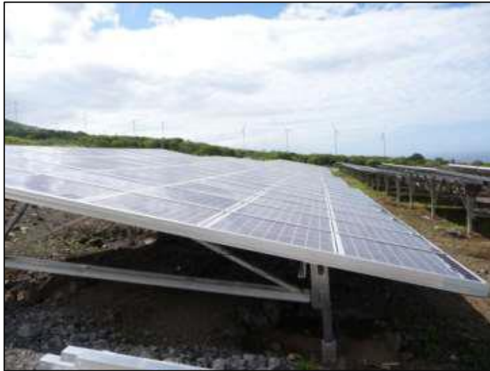
Figure 14: Example of a fixed mounted PV System.
