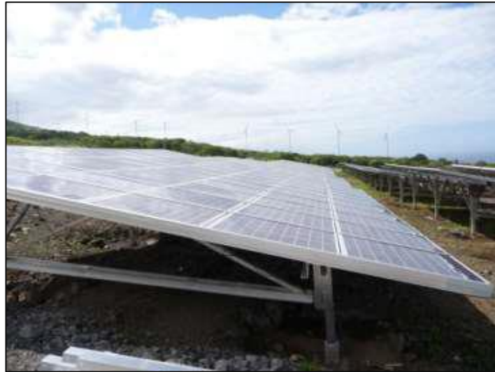
Figure 13: EXAMPLE OF A FIXED MOUNTED PV SYSTEM.
