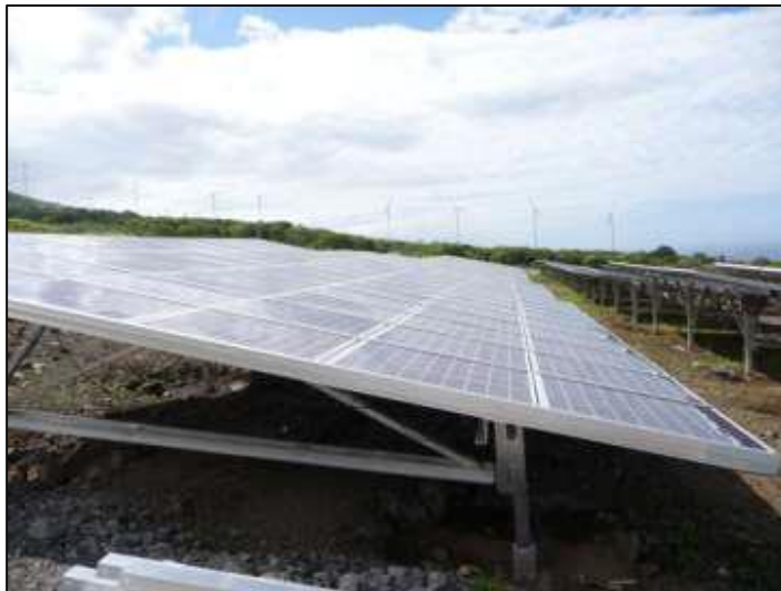
Figure 14: EXAMPLE OF A FIXED MOUNTED PV SYSTEM.
