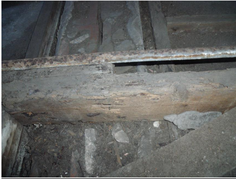
Figure 2-Truss Tie beam damaged by wood borer
