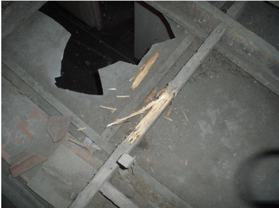
Figure 5- Wood borer damage on ceiling brandering
