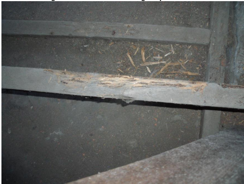
Figure 3- Ceiling joist damaged by wood borer
