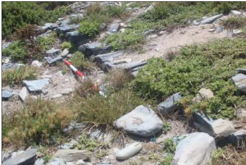
Figure 8: One course of revetment wall exposed, the wall appears to be buried by stones and soil wash.
