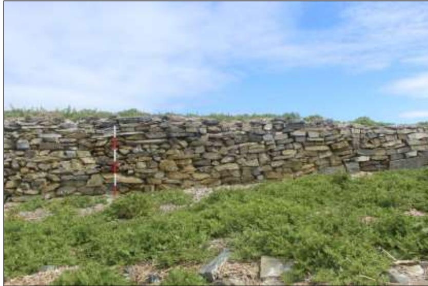
Figure 1: Sections of the wall that are standing and intact will be preserved
