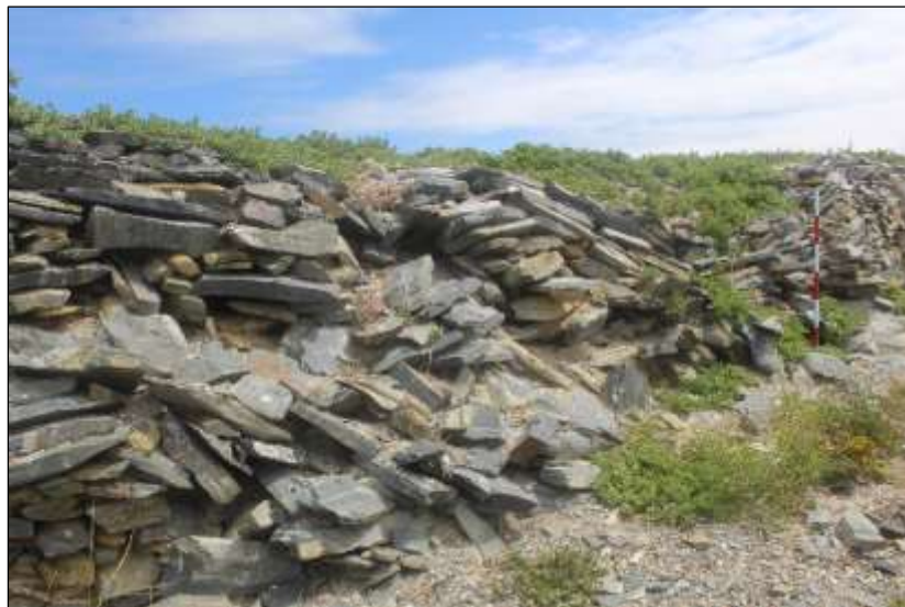
Figure 2: Partially collapsed sections will be restored using the same material which has been displaced
