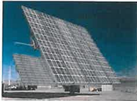
Figure 2: Typical CPV Unit
