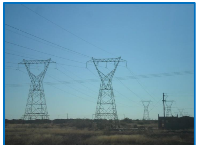
Plate 3: View of Eskom powerlines
