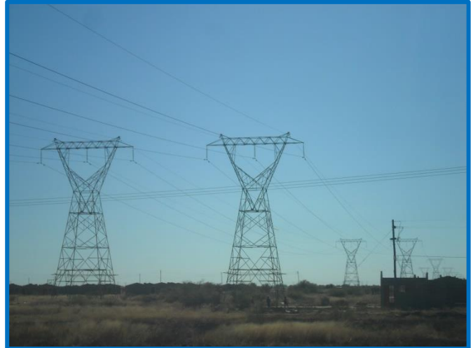
Plate 3: View of Eskom powerlines
