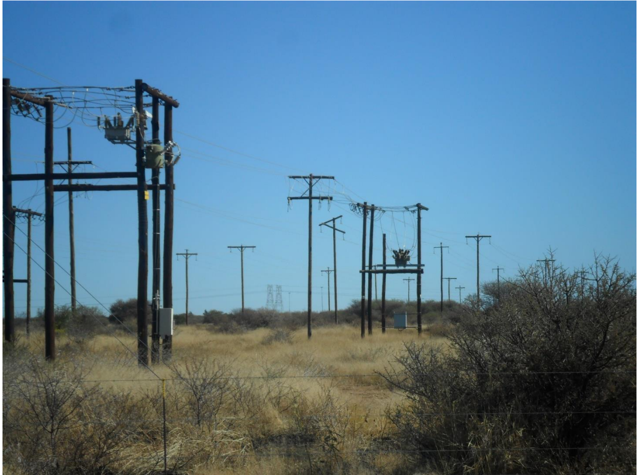
Plate 1: View of the four (4) powerlines located adjacent to the northern boundary of the development area
