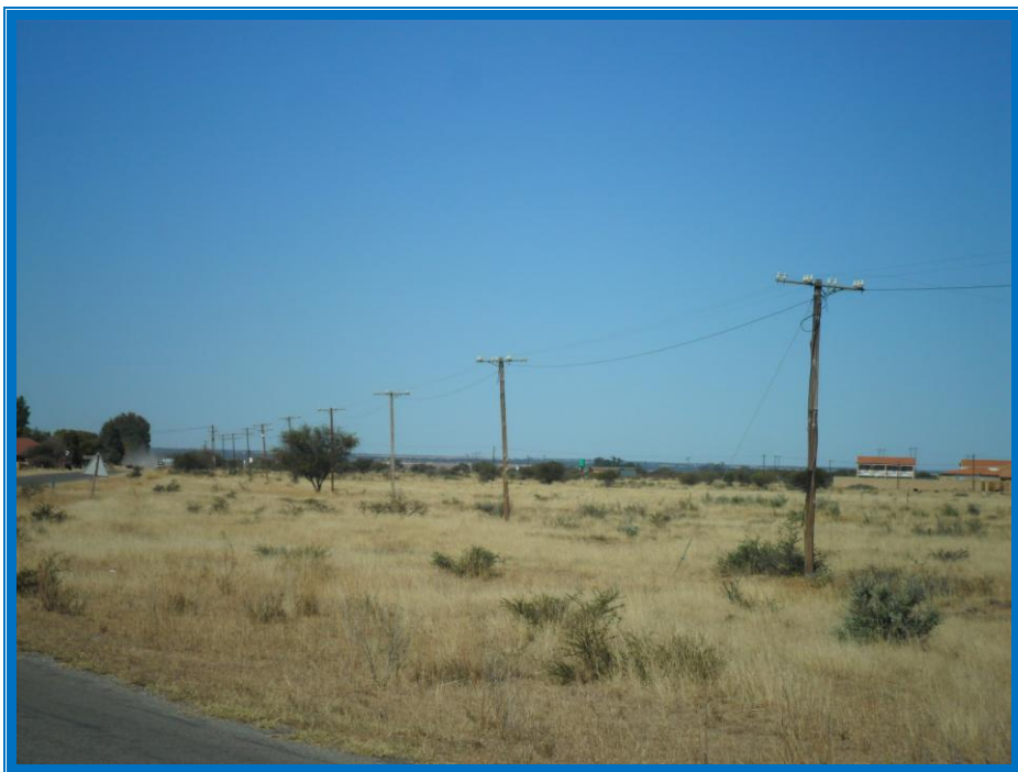
Plate 2: View of Telkom telephone lines locate along the eastern boundary of the northern portion of Amalia Extension 5
