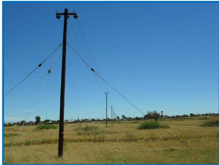
Plate 8: Eskom powerline to Lebaleng
