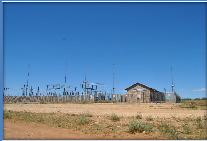
Plate 5: View of existing Naledi Main Substation
