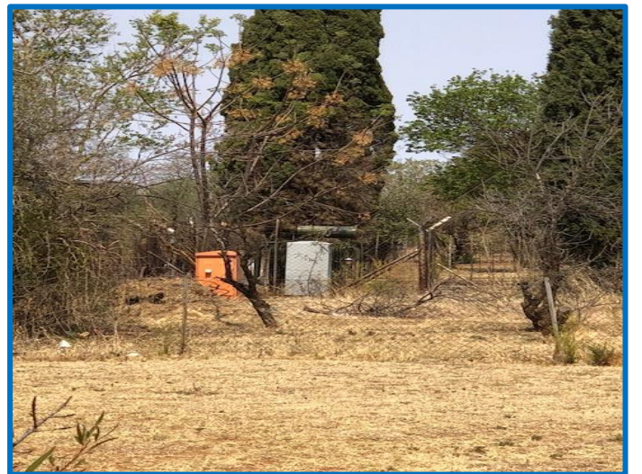
Plate 6: Existing sub-station infrastructure
