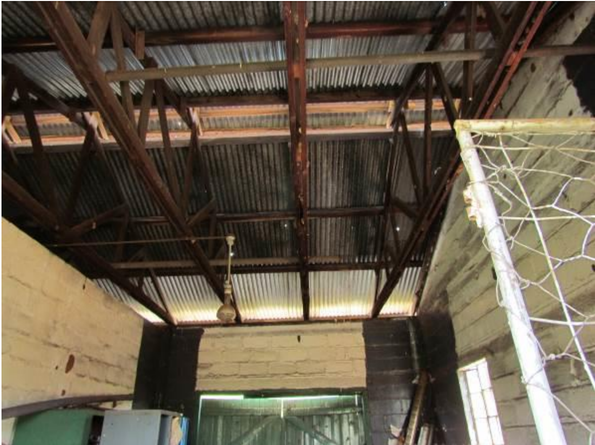
Figure 11: Interior view of substation structure
