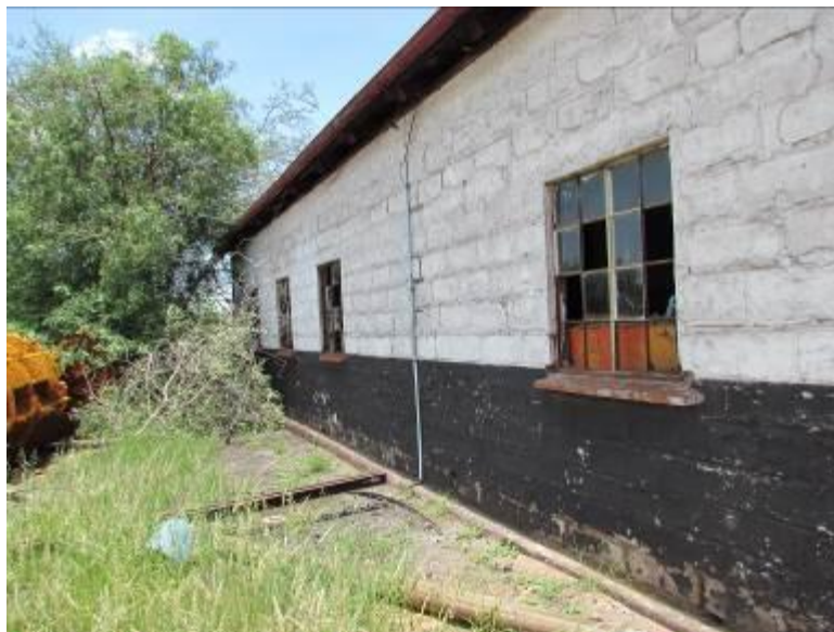
Figure 10: Side view of substation structure
