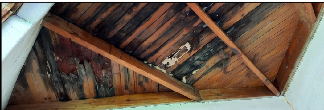
Rotting to the roof timber.
