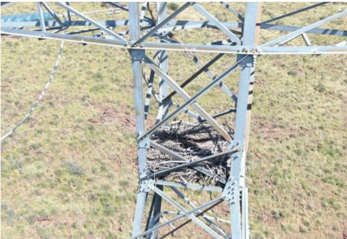
Figure 4: A Verreux's Eagle nest in a high voltage line at the project site.
