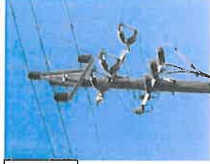
Figure 11: Typical 22KV single Powerline
