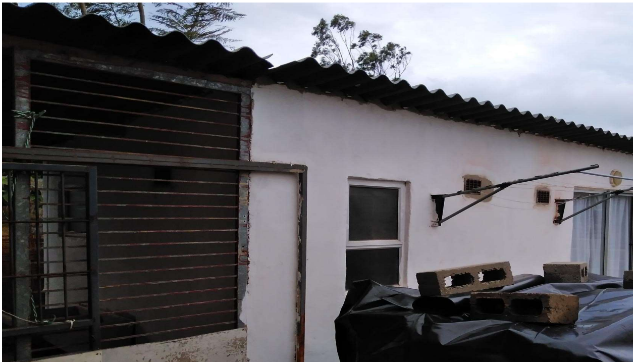
W. ELEVATION - NEW PRIV GYM (OLD ROOF IN /ILLEGAL BUILDING )
