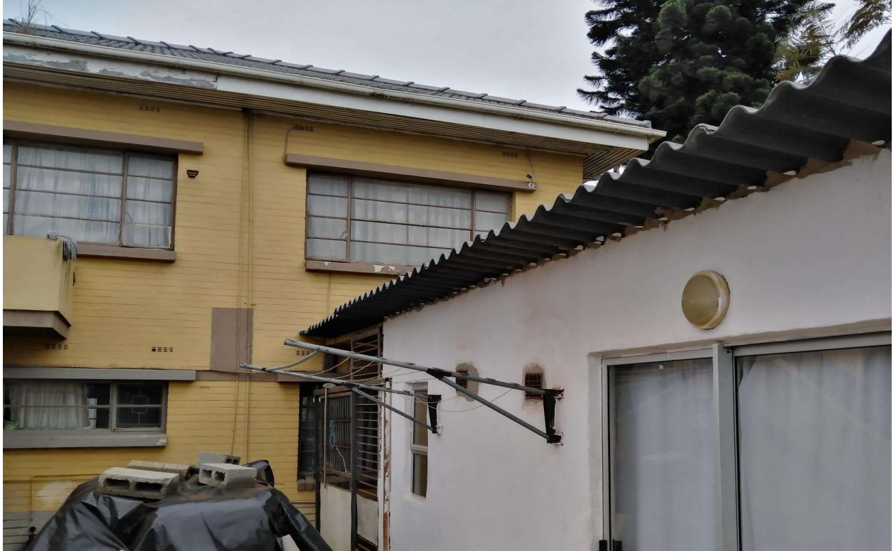
EX DWELLING & NEW PRIV GYM (ILLEGAL BUILDING - OLD ROOF IN) - S. ELEVATION
