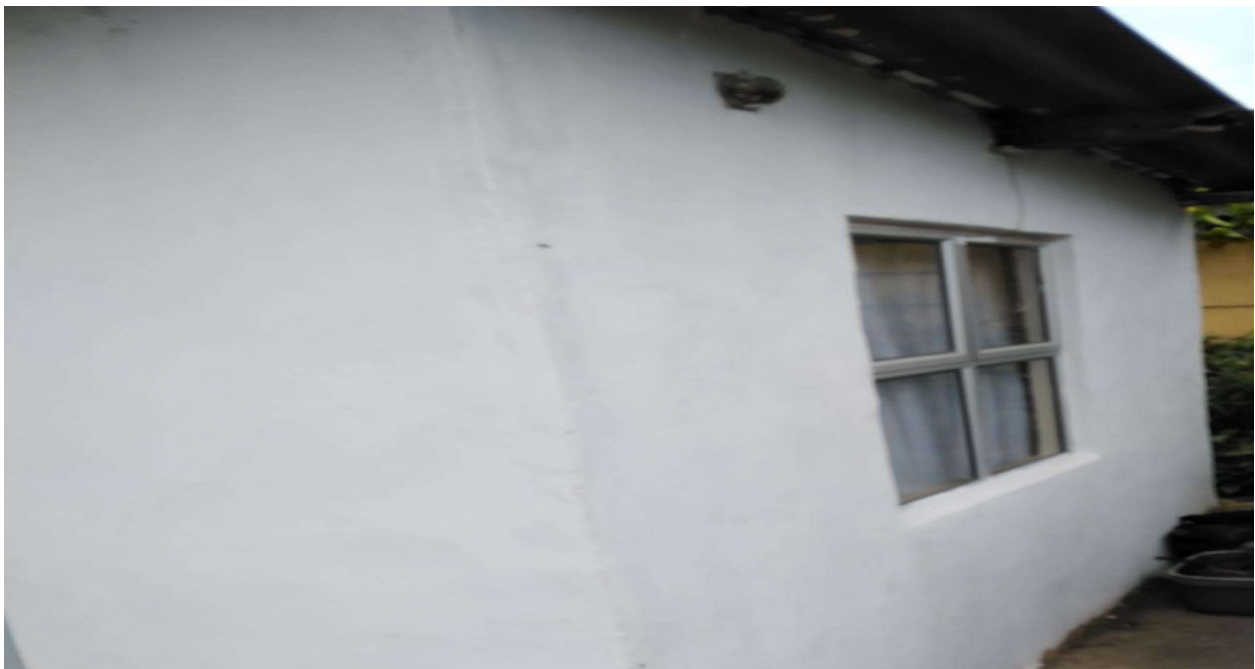
NEW PRIV GYM - S. ELEVATION (ILLEGAL BUILDING - OLD ROOF IN)
