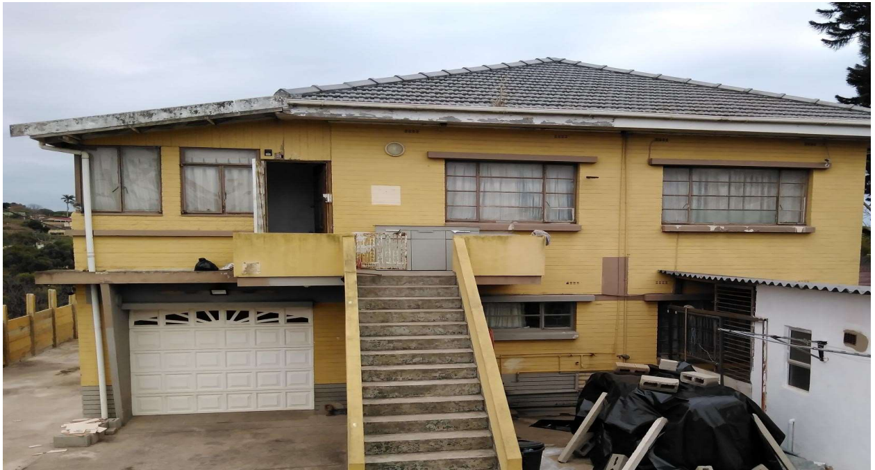
EX DWELLING & NEW PRIV GYM (ILLEGAL BUILDING - OLD ROOF IN) - S. ELEVATION
