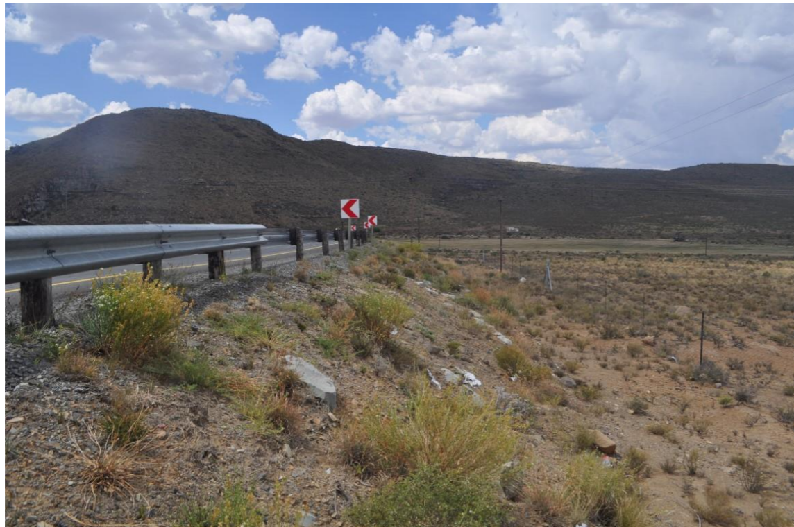
Road has been lifted / Guardrails / No Access to "road" shown on Google Earth
