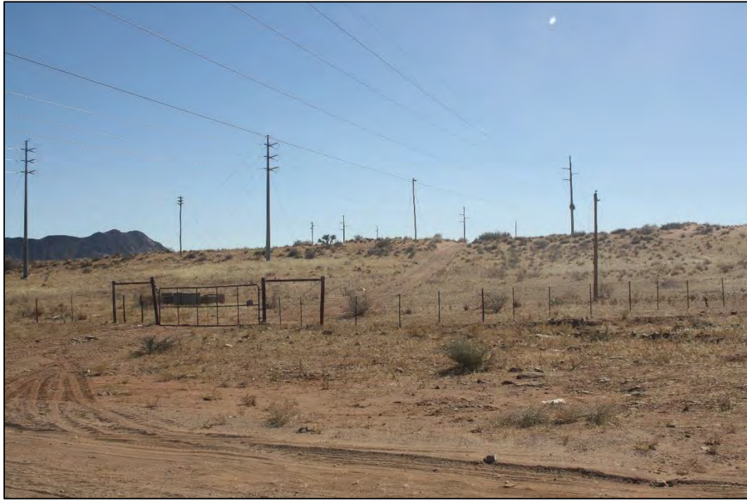
Figure 22: View of power lines connecting to Paulputs substation.
