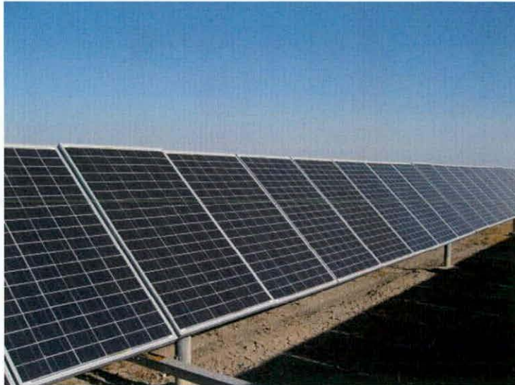
Figure 2.2: Photograph illustrating photovoltaic panels
