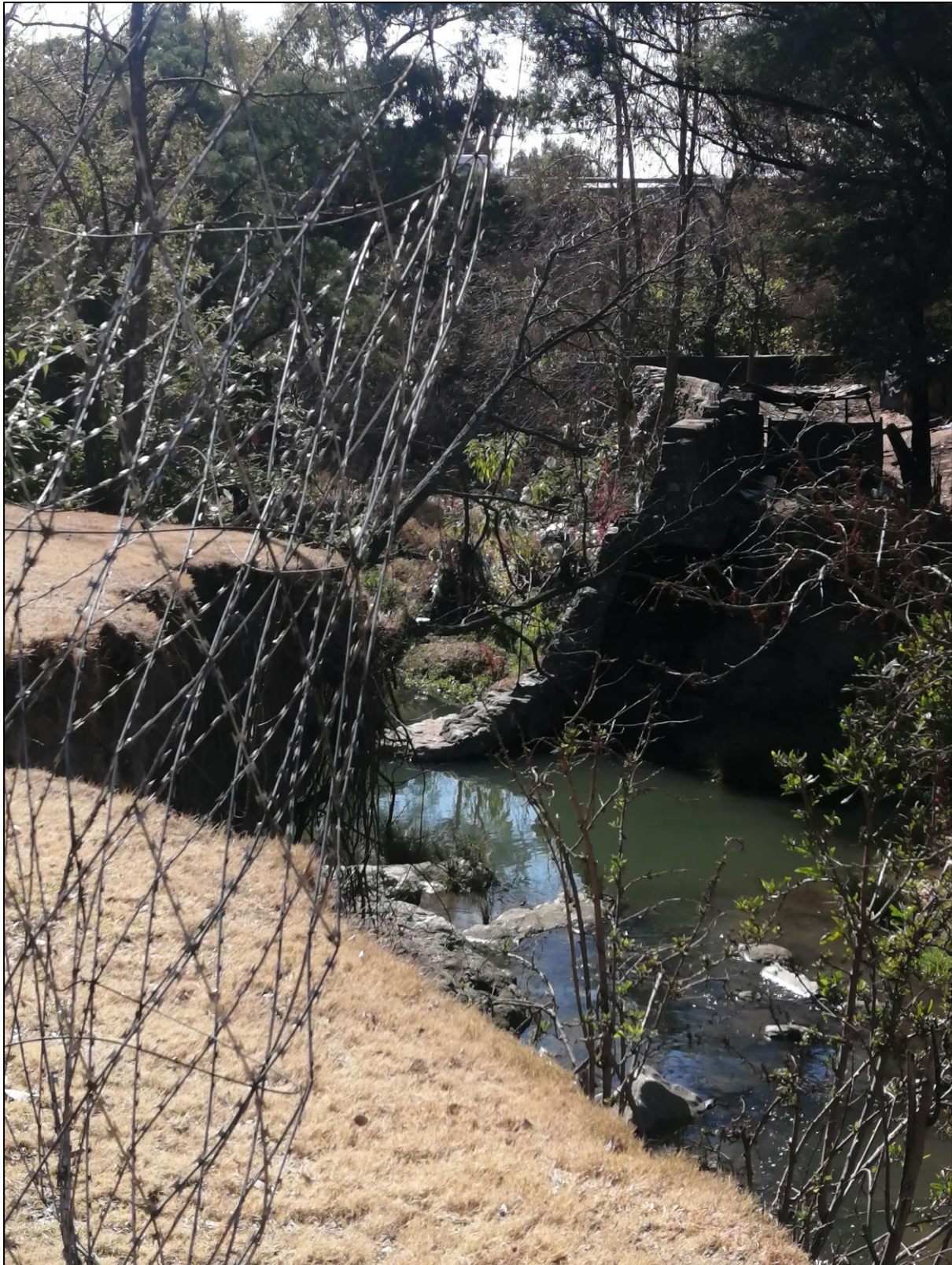
Figure 7-6: Impacts to the geomorphology – erosion and incision as a result of the stormwater runoff intensities
