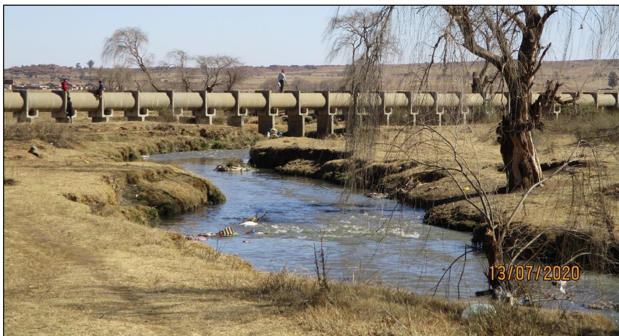
Figure 10: Sewage discharge within the wetland – damaged and deteriorated pipeline
