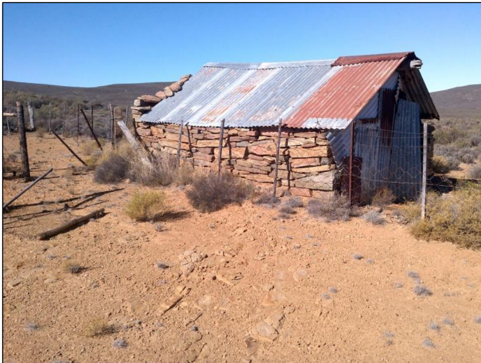
Figure 53: View of the modified stone walling cottage (BV_SW12) situated within the route proposed for the upgrade of the access roads.
