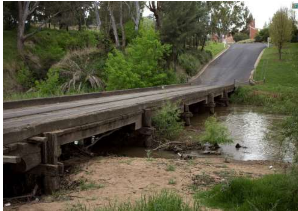
Figure 5: Images above showing a low-level bridge design, which would be inundated with water flow during rains
