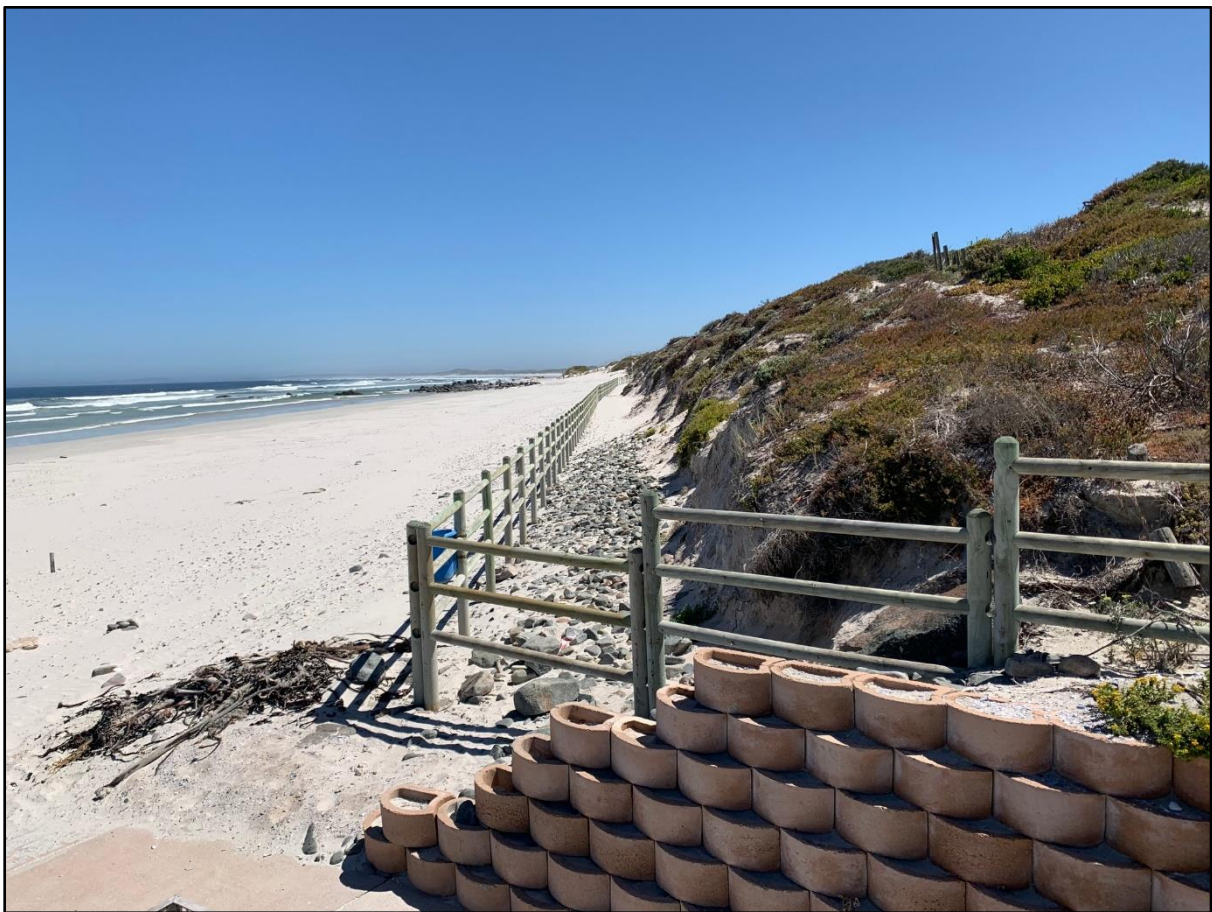
Figure 10. Image showing rip rap on dune toe to the north of cable landing point, where “Alternative 2” is proposed.
