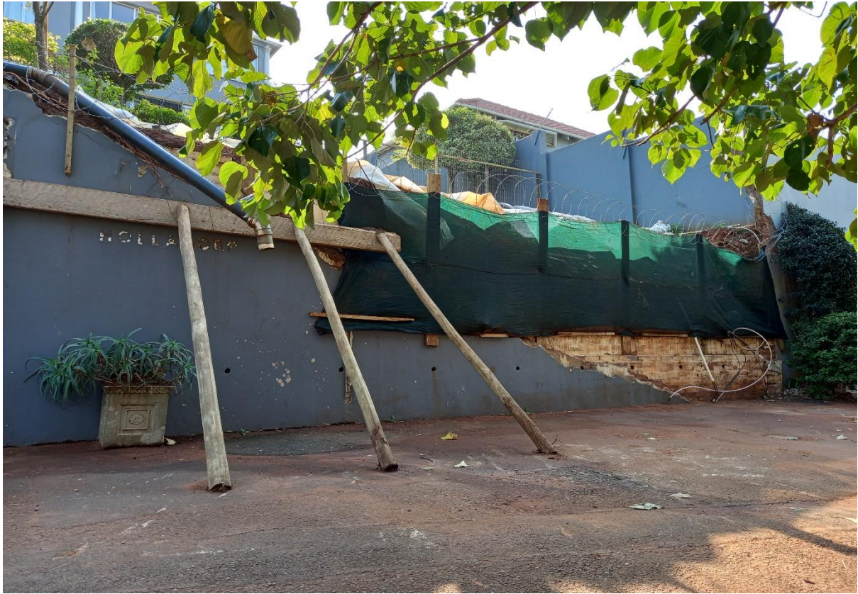
FRONT ELEVATION OF COLLAPSED RETAINING WALL
