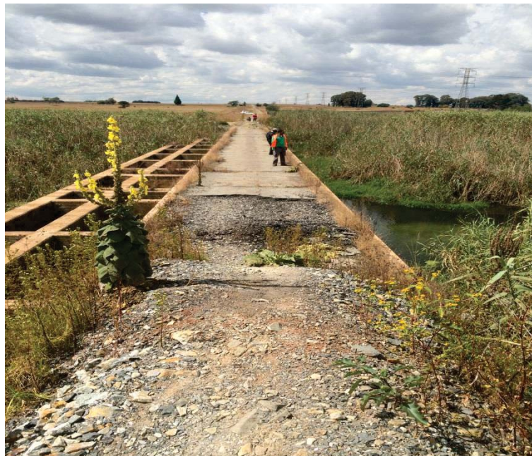
Figure 6-11: Picture taken west of Largo Site 4 showing the proposed pipeline route from Largo Site 4 to the proposed HDS Plant
