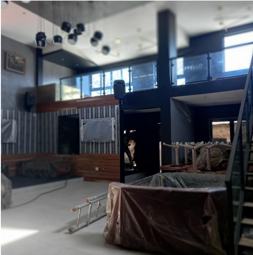
Image 4 – Damaged unstable wooden floors removed at first floor to make double volume and ground floor is replaced with concrete floors.
