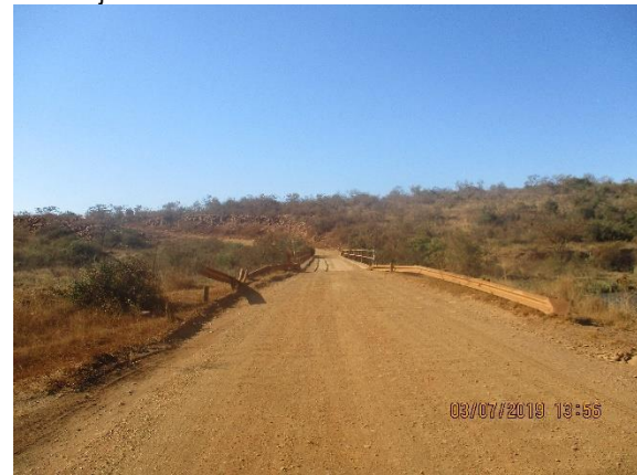
Photo 4: View of the existing single lane bridge over the Mozana River crossing point.
