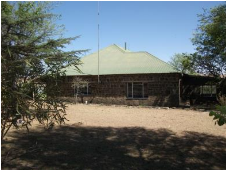
Figure 68: The main residence (FC02.1) in FCO2 was constructed with dressed dolerite stone and is a multi-roomed structure with steel window frames which was covered with a pitched corrugated iron roof (above).
