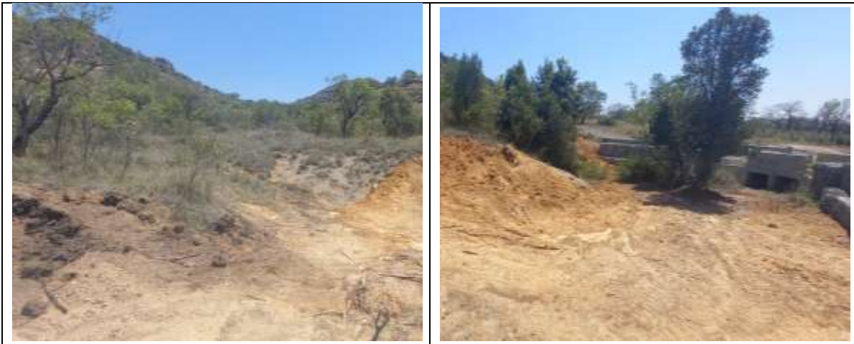
Plate 3.20: Upstream incised alluvial channel of W1.10, with cleared area, material fill and culvert crossing
