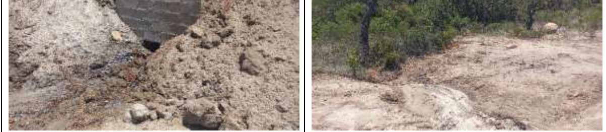
Plate 3.26: Small culvert, creating a knick point and downstream erosion and sedimentation.
