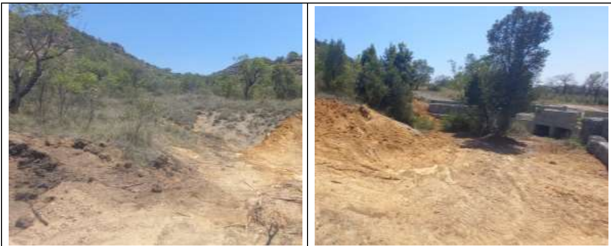
Plate 3.15: Upstream incised alluvial channel of W1.10, with cleared area, material fill and culvert crossing
