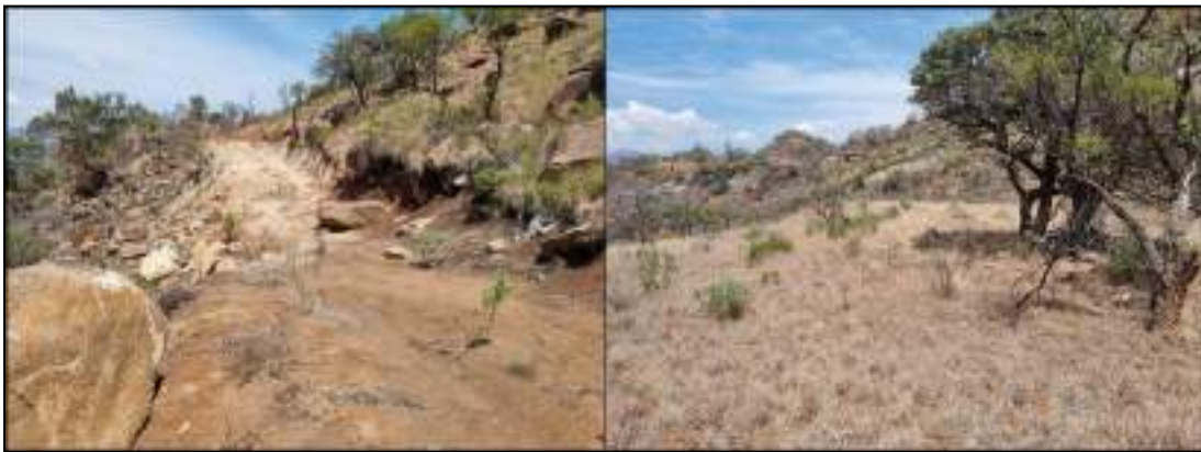
Figure 4-2: View of an eroded access road and general surroundings in the project area.
