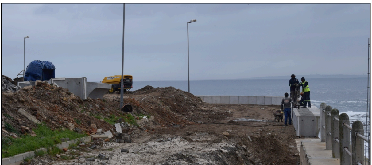
Photograph 8: Current improvements to the Promenade precinct 2 sea wall and landscaping, 2017 The brine discharge pipeline is proposed to be aligned along the seawall.
