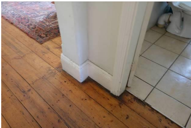
Fig. 40_Original wooden skirtings and Oregon pine floor boards along the passage and lounge area (Source: tsica heritage consultants, 22.09.2020)
