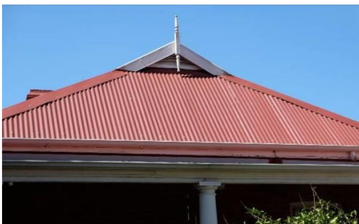
Fig. 22_ Roofing detail with air vent and fine detailing (Source: tsica heritage consultants, 22.09.2020)
