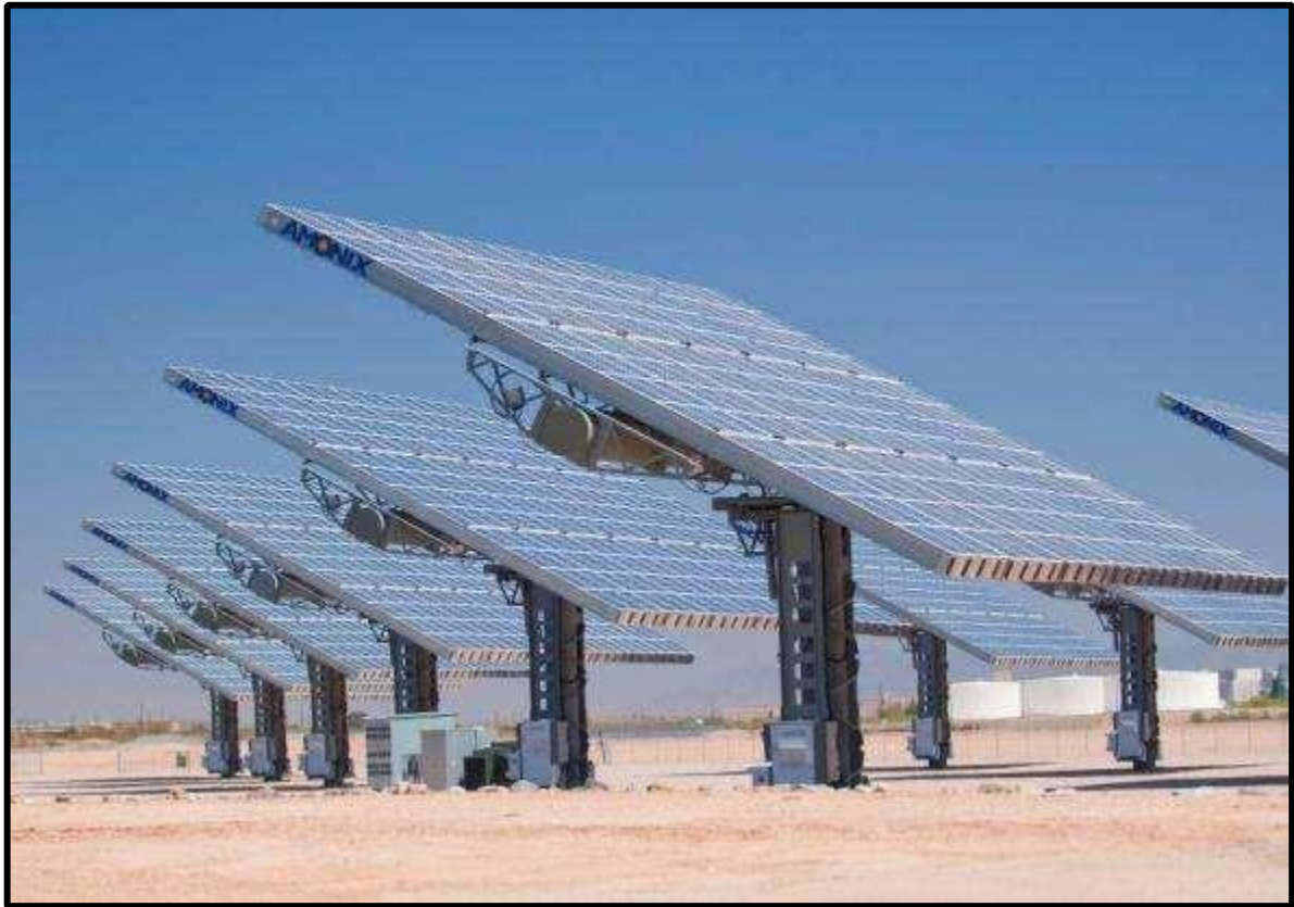
Figure 1.4: Illustration of a tracking solar energy facility (Courtesy of Amonix™)
