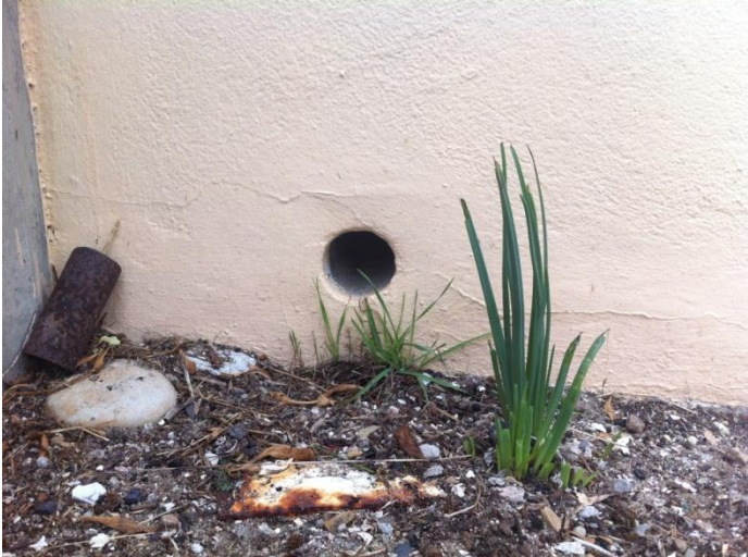
Detail of rust and vegetation
