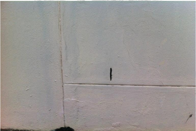
Slips in the wall
