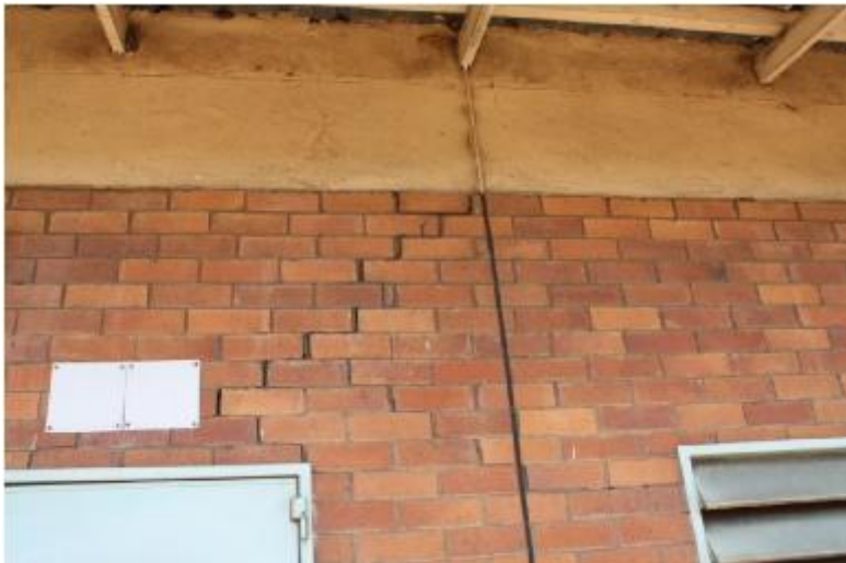
Figure 8: Example of blast induced damage.
