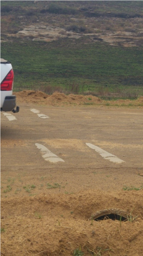
Photo 4: Poor Drainage on Main Access Road D638
