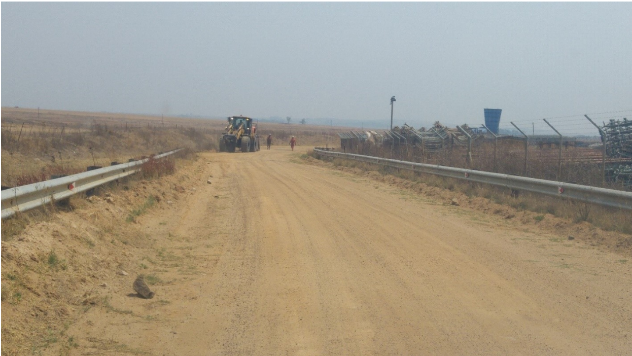
Photo 7: Secondary Access Road D638 encroached by mine complex
