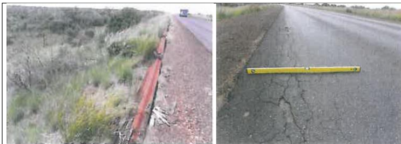
Poorly maintained guardrail/s
