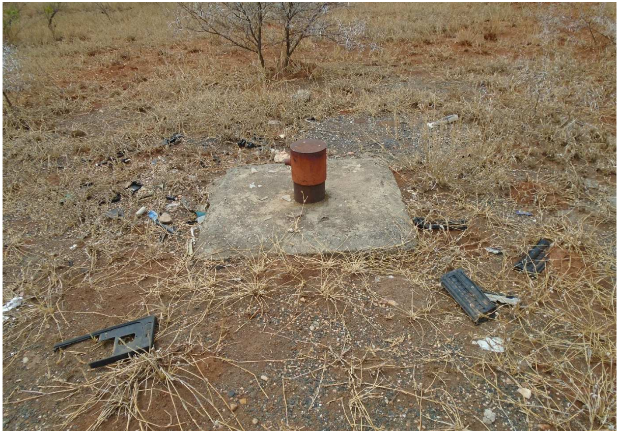
Figure 8: A municipality borehole on site
