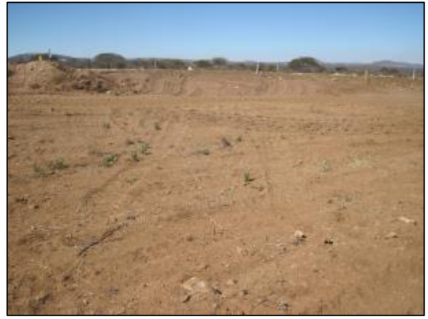
Figure 29: View of the earth moving activities from the adjacent N1 bypass development.
