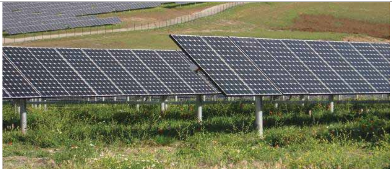
Figure 1: Fixed tilt PV array
