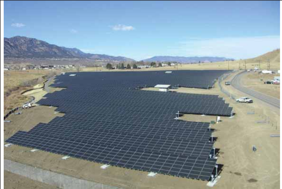
A 2-megawatt, ground mounted PV array occupies the site of a former landfill at Ft. Carson, Colorado, USA (Source: www.wapa.gov )
