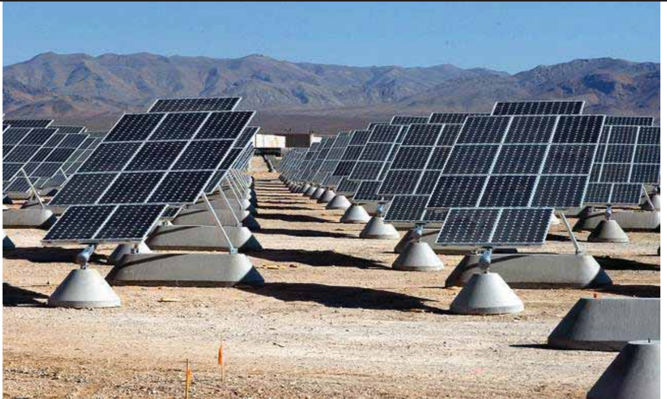
Figure 2: Tracking PV array
