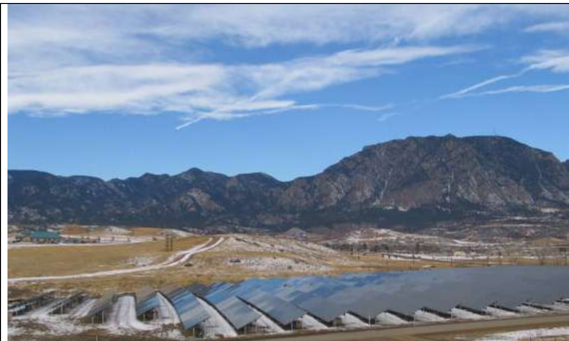
A 2-megawatt, ground mounted PV array occupies the site of a former landfill at Ft. Carson, Colorado, USA (Source: www.wapa.gov )
