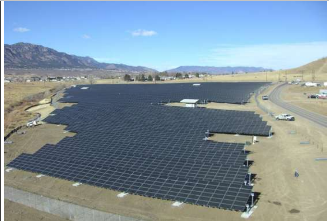
A 2-megawatt, ground mounted PV array occupies the site of a former landfill at Ft. Carson, Colorado, USA (Source: www.wapa.gov )
