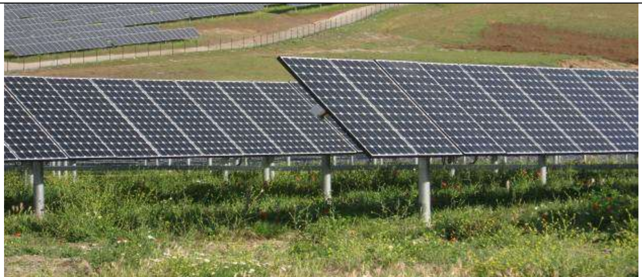
Figure 1: Fixed tilt PV array
