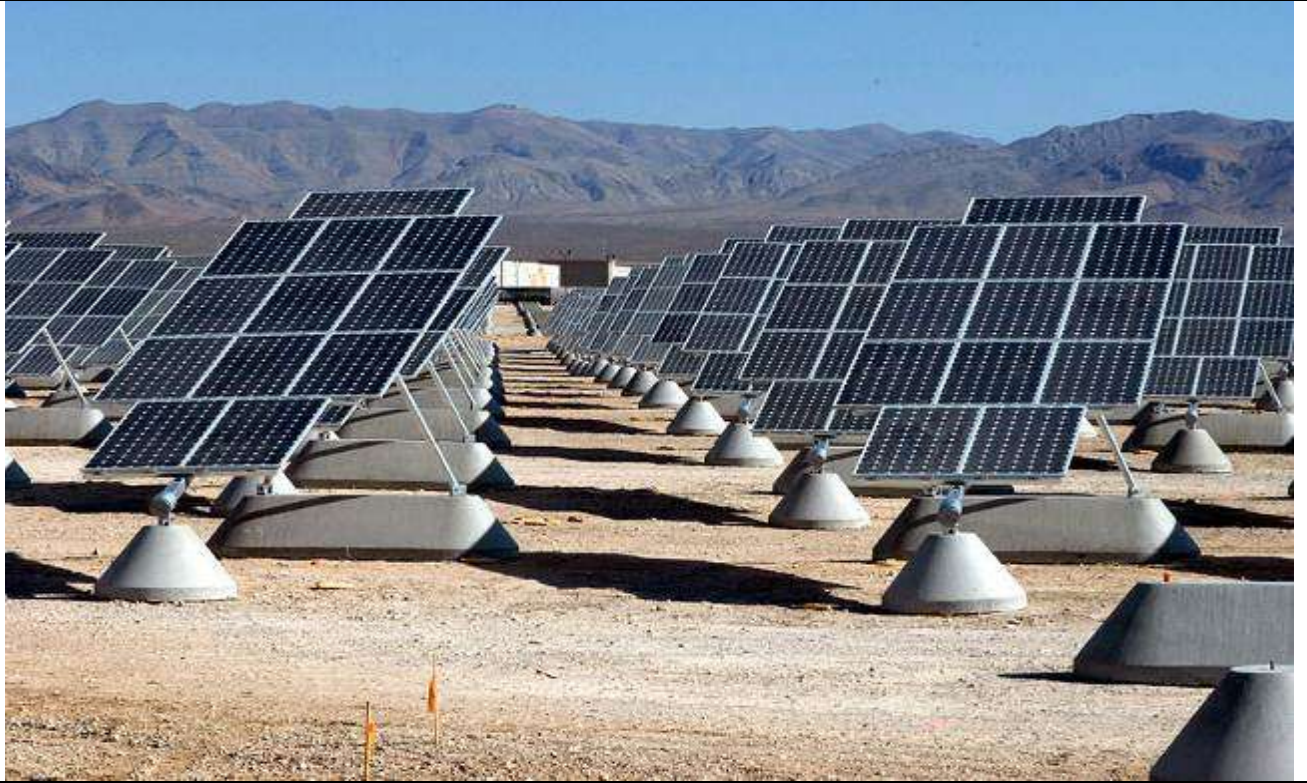
Figure 2: Tracking PV array
