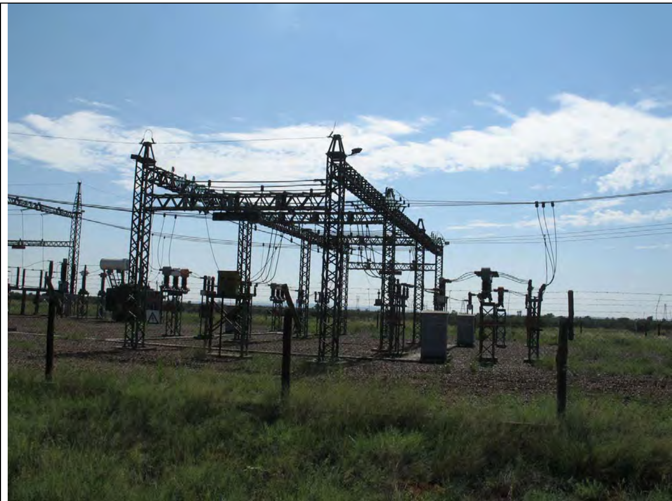
Figure 3-4: Existing Dougnor substation within the farm Adams 328.
