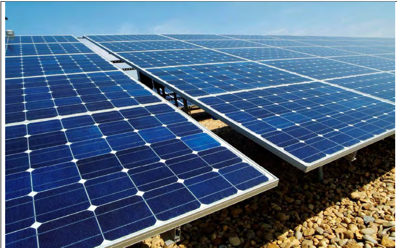
Figure 3-1: Fixed tilt PV array (sourced http://explow.com/solar_panel )
