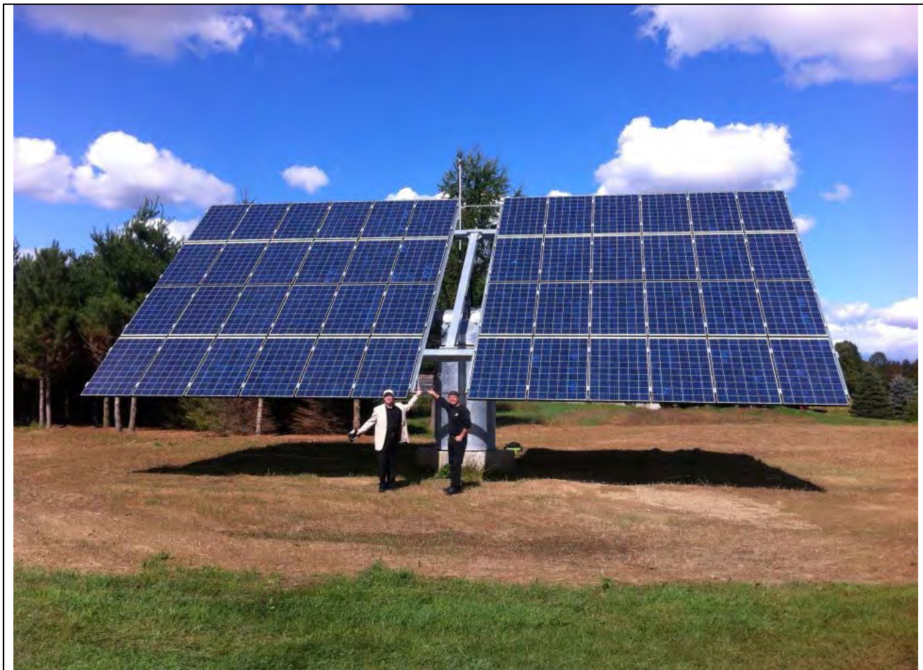
Figure 3-2: Tracking PV array (sourced http://solarblog.ca )
