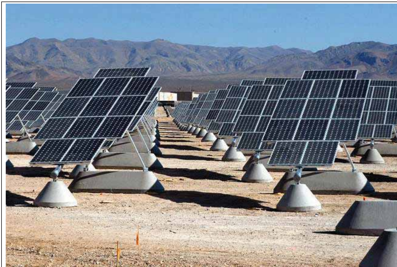
Figure 3-2: Tracking PV array
