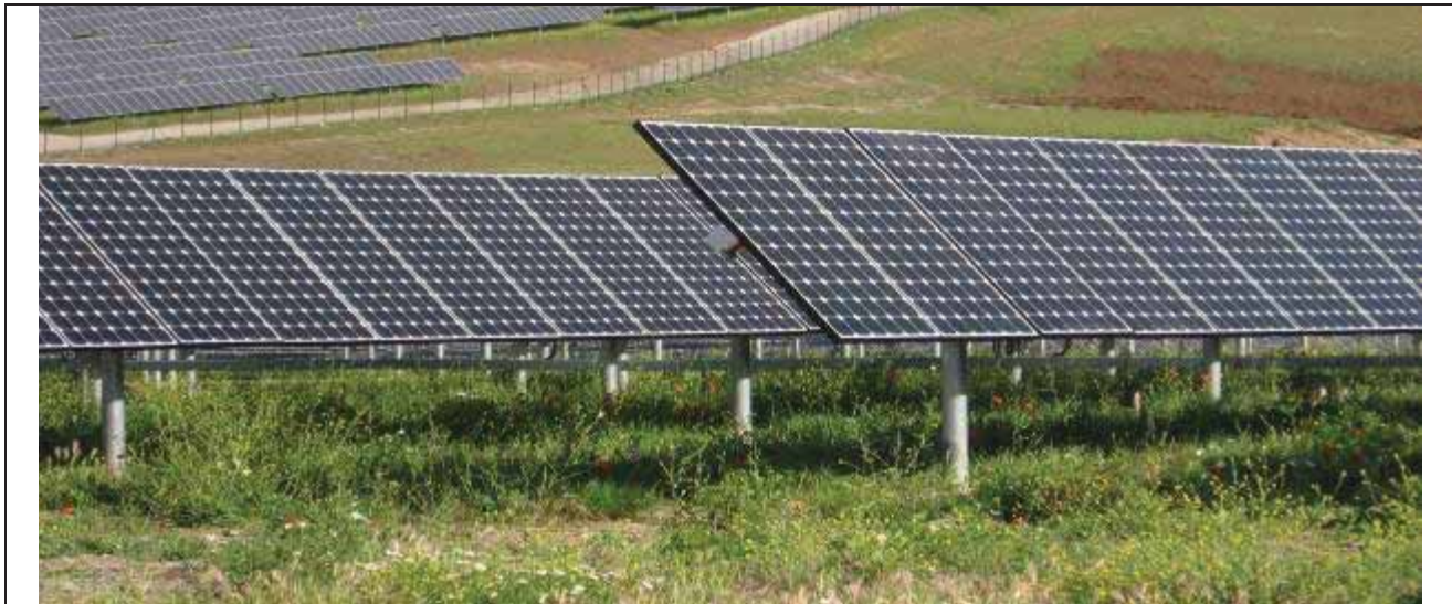
Figure 3-1: Fixed tilt PV array
