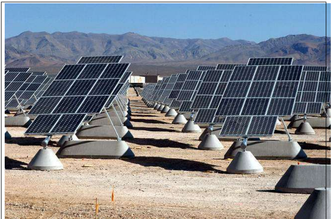
Figure 3-2: Tracking PV array
