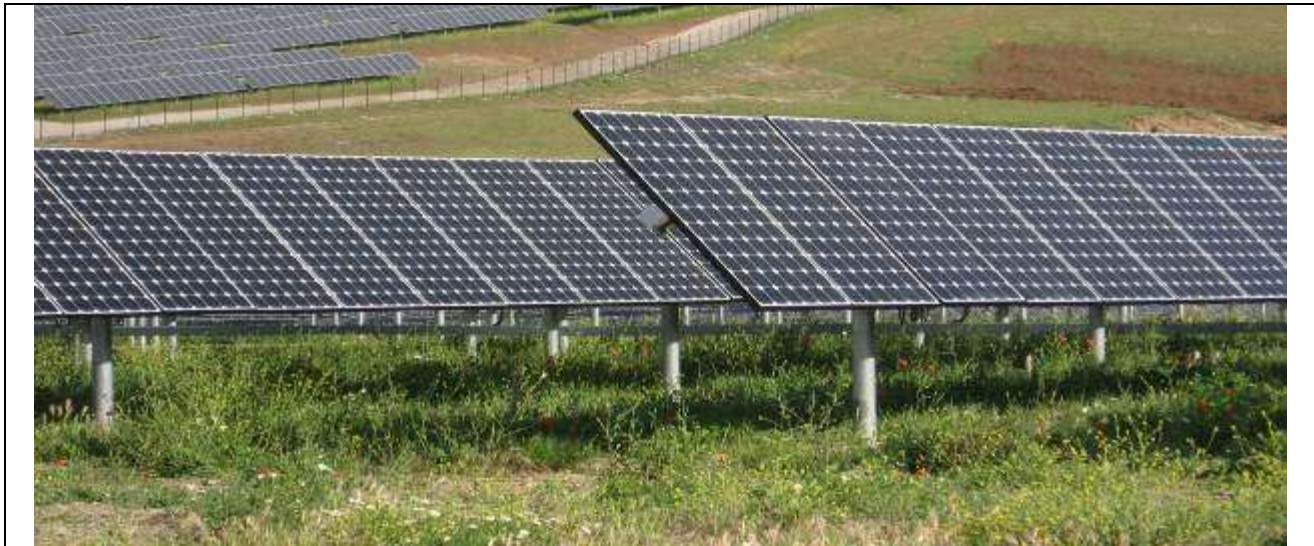
Figure 3-1: Fixed tilt PV array
