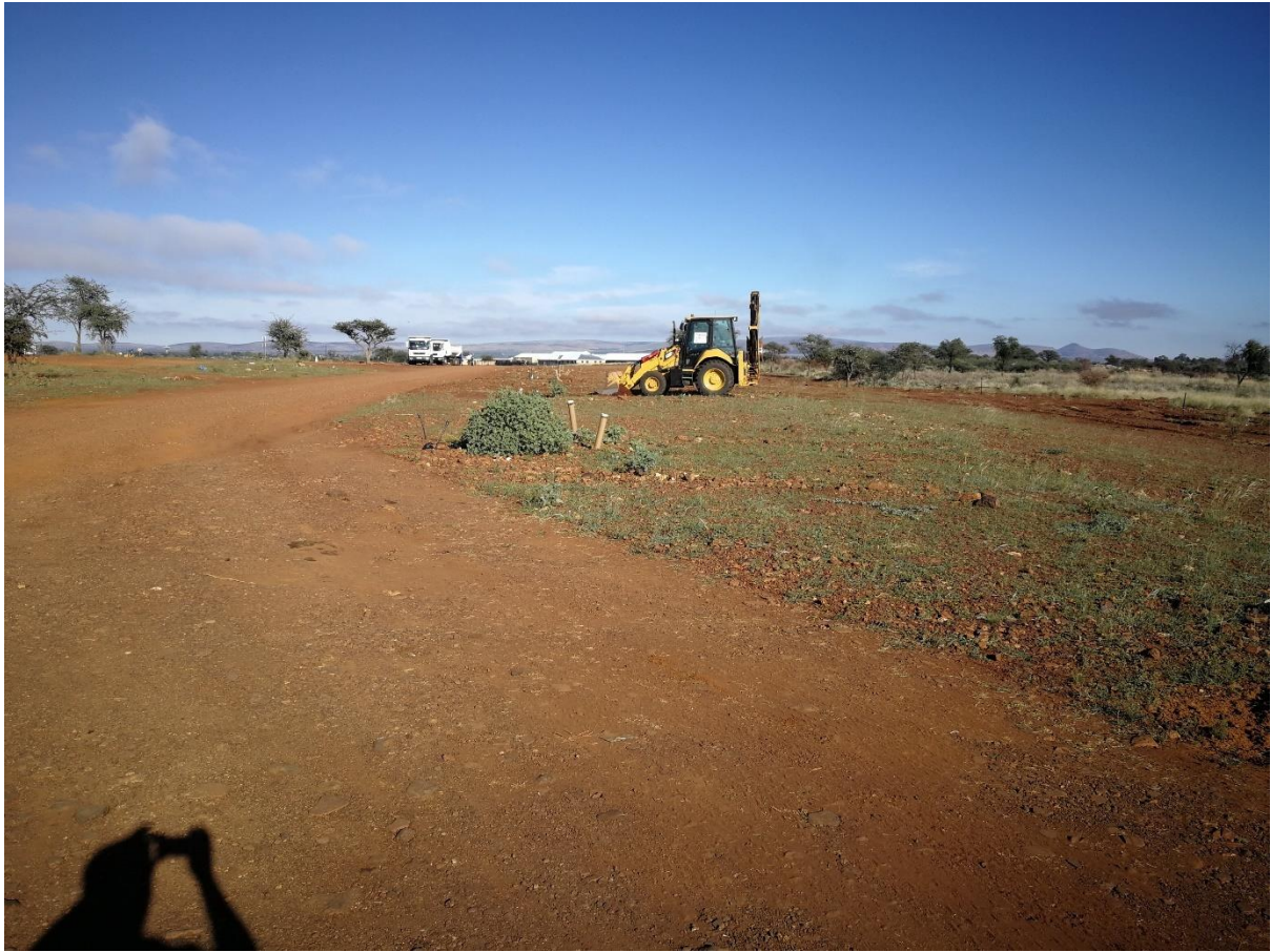
Photo 2: Earthworks pertaining to Phase 1 of Wrenchville Low-Cost Housing Development adjacent to concerned property. Direction: West
