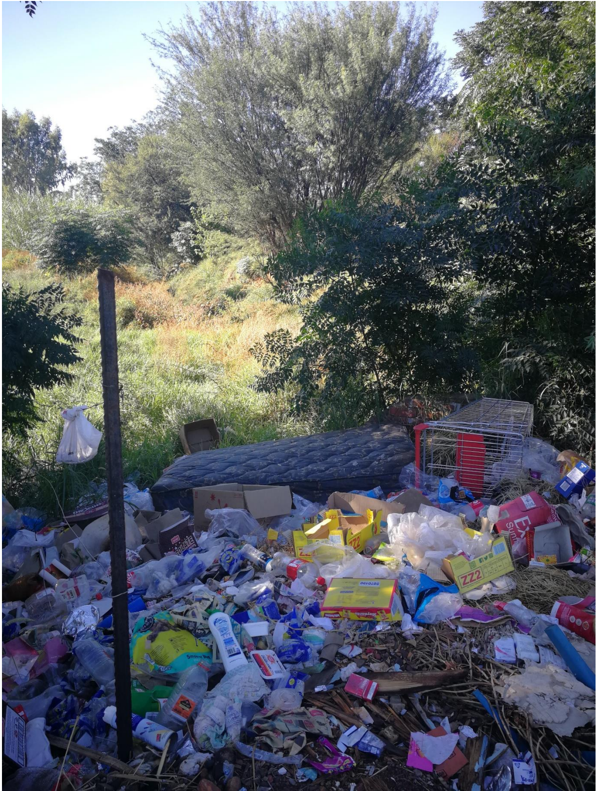
Photo 50: D41L-02299 culvert crossing underneath Mossie Street in Wrenchville. Severely overgrown and polluted. Direction: East.
