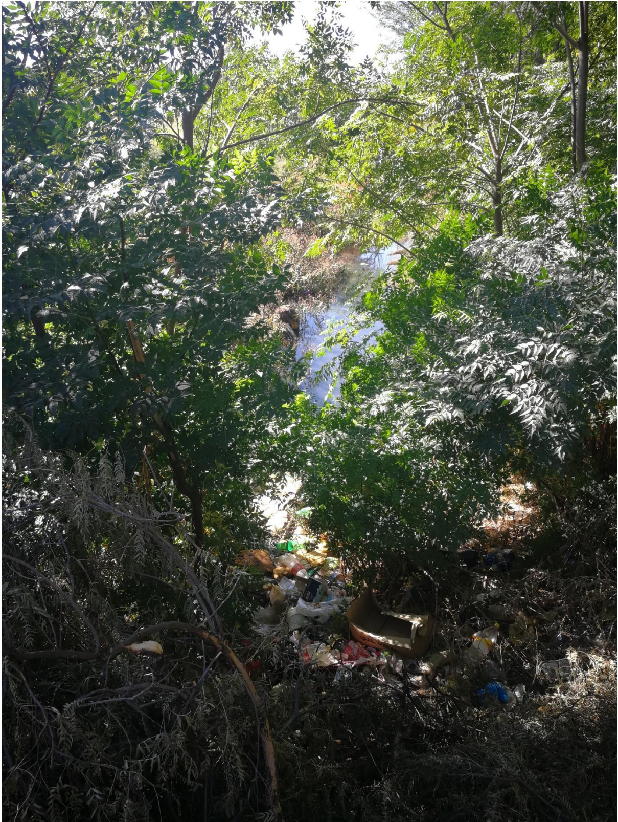
Photo 51: D41L-02299 culvert crossing underneath Mossie Street in Wrenchville. Severely overgrown and polluted. Direction: East.
