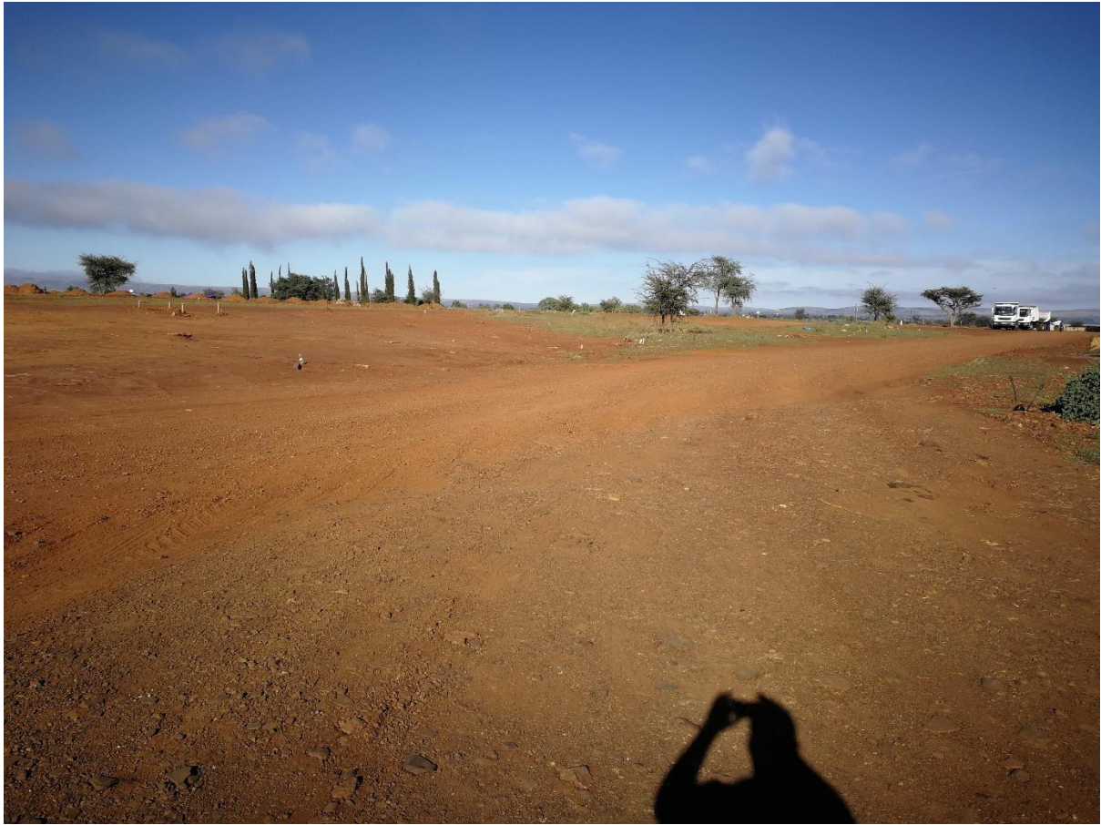
Photo 3: Earthworks pertaining to Phase 1 of Wrenchville Low-Cost Housing Development adjacent to concerned property. Existing graveyard visible in the background. Direction: South.
