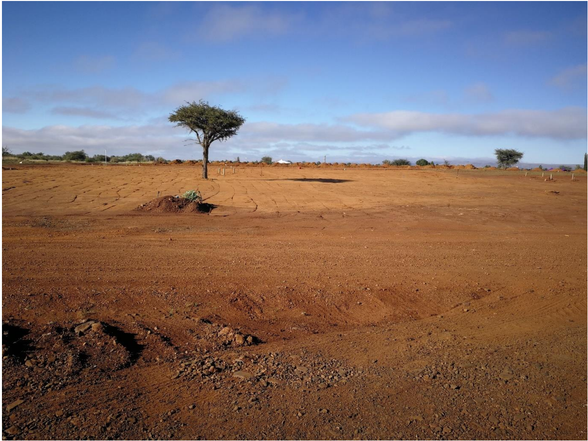
Photo 1: Earthworks pertaining to Phase 1 of Wrenchville Low-Cost Housing Development adjacent to concerned property. Direction: South
