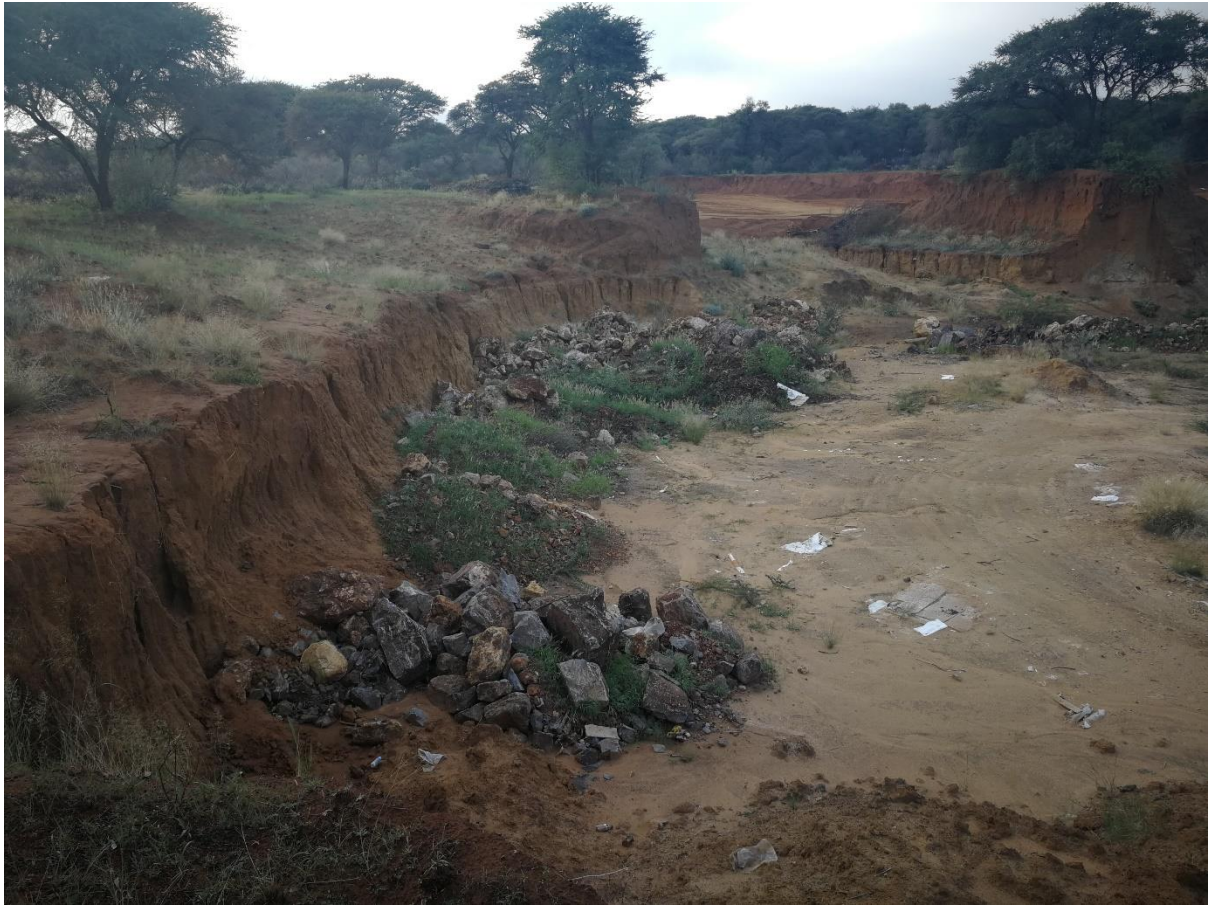
Photo 17: Sand quarry with rubble piles situated in the North-Eastern corner of the proposed development area. Situated within the concerned stream channel and associated Riparian Area. Natural Kuruman Thornveld Vegetation. Direction: East
