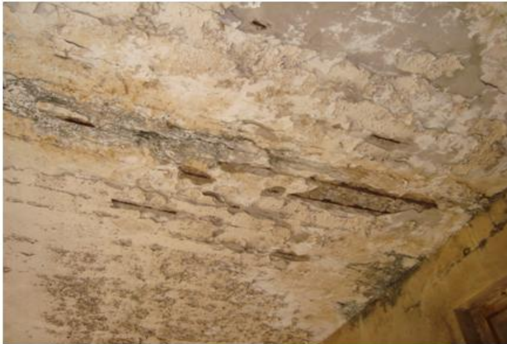
Figure 1 Spalling rebar at bottom of slab over East entrance veranda
