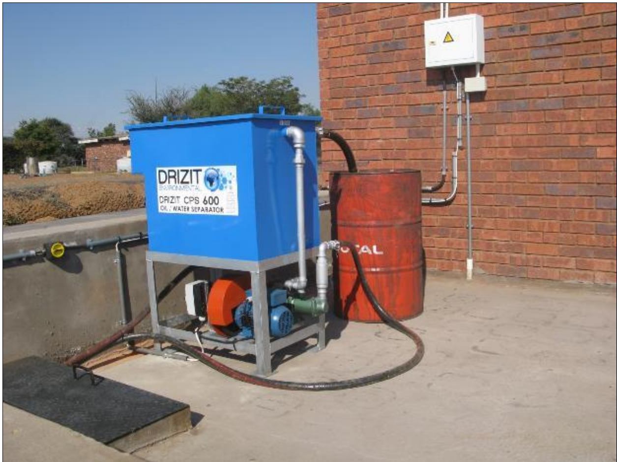
Figure 2-10: Storm water collection sump and treatment Black Rock hazardous waste storage facility
