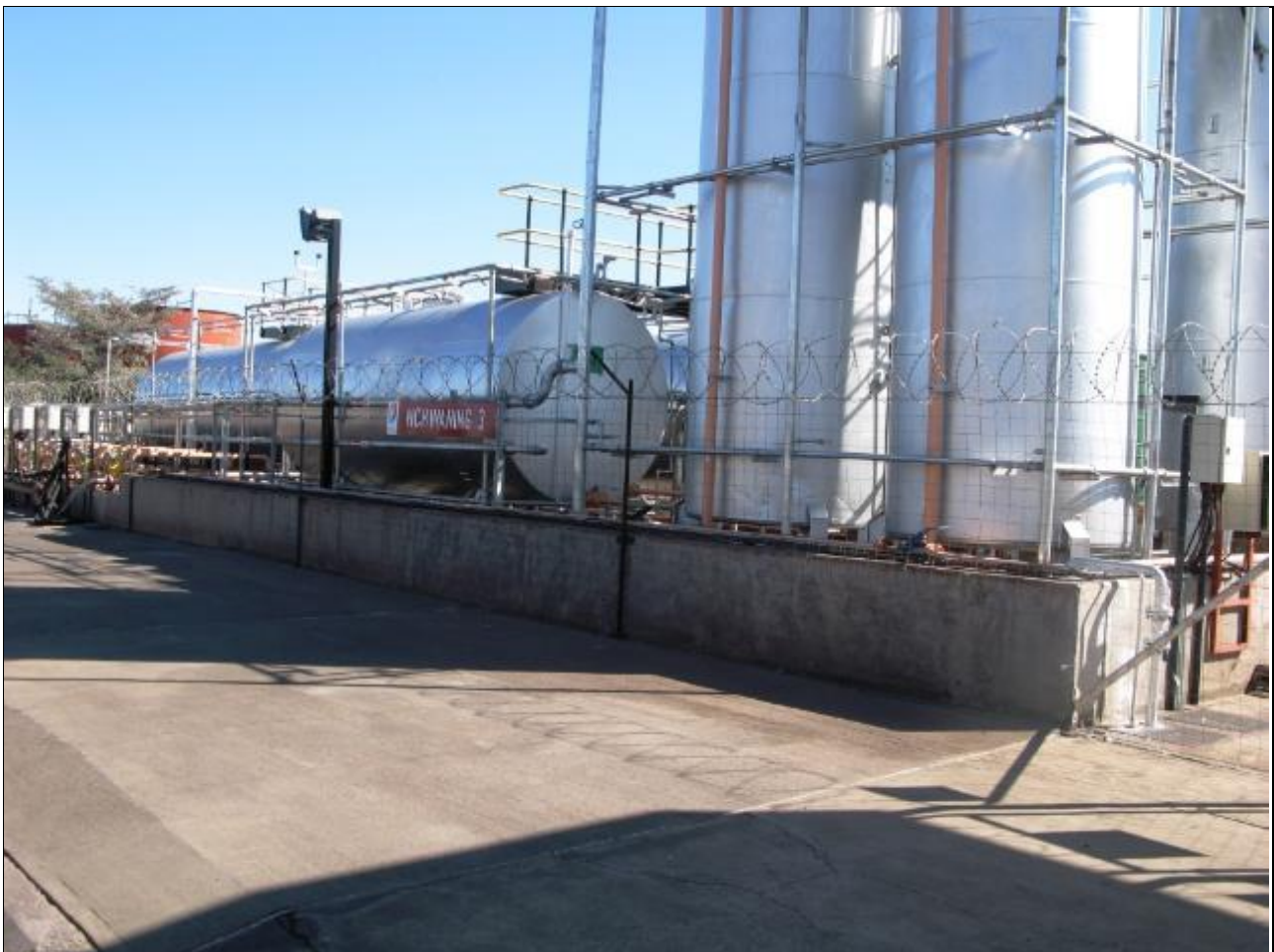
Figure 2-7: Example of existing bunded fuel storage at Nchwaning III
