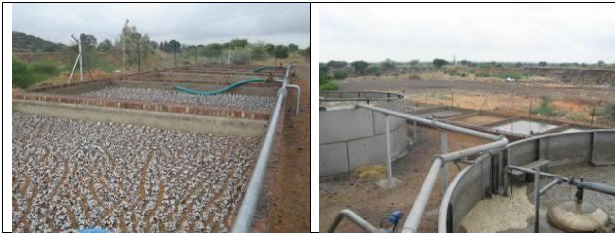
Sludge Drying Beds Maturation Tanks Figure 2-6: Photographs of existing Black Rock SWTP
