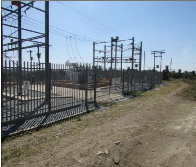
Fig.3: View of existing Aloe Substation.
