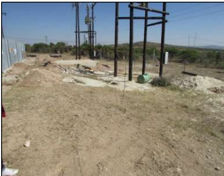
Fig.4: View of expansion area (for new Transformer) next to existing Aloe Substation. It is in this area that unknown burial was uncovered.
