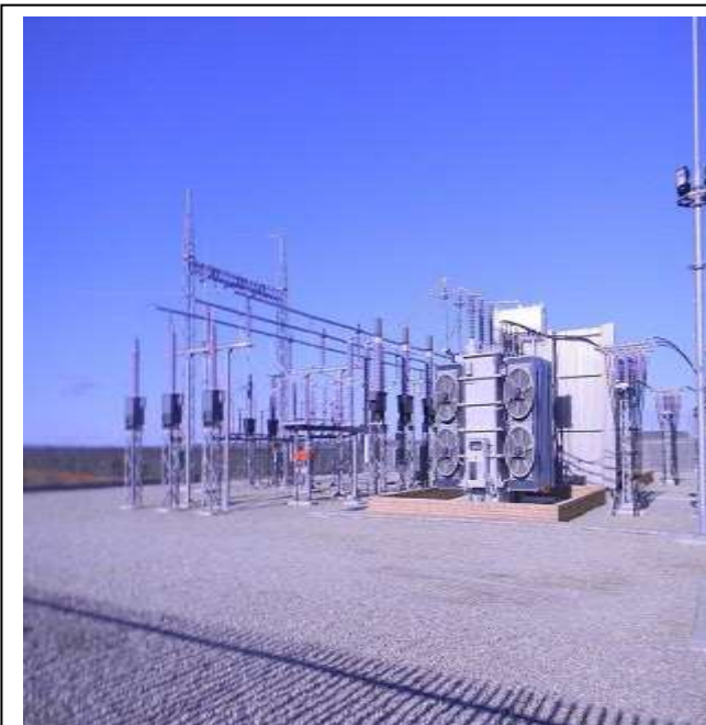
Figure 7.4: Substation (Eskom Sere Wind Facility)
