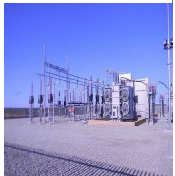
Figure 7.4: Substation (Eskom Sere Wind Facility)
